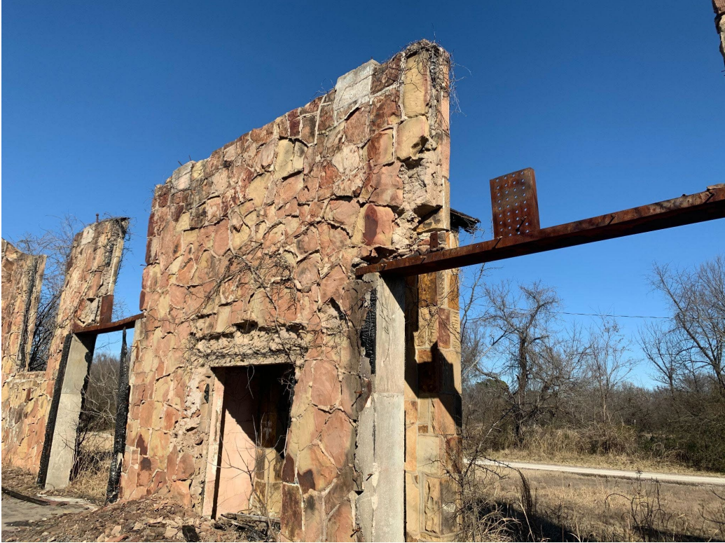
Figure 2 - Interior view of the east wall within the north section of the building.
